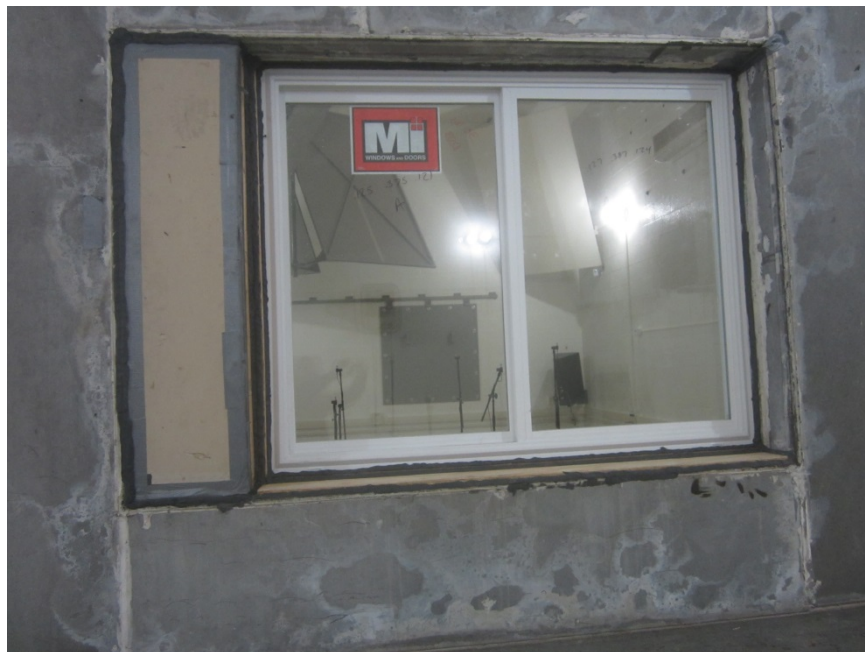
Source Room View of Installed Specimen
