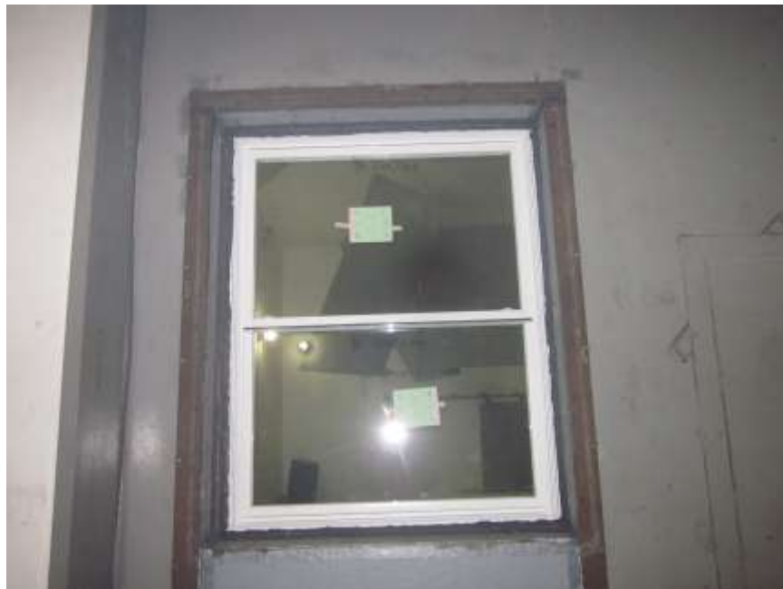
Source Room View of Installed Test Specimen
