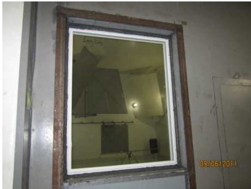
Source Room View of Installed Test Specimen
