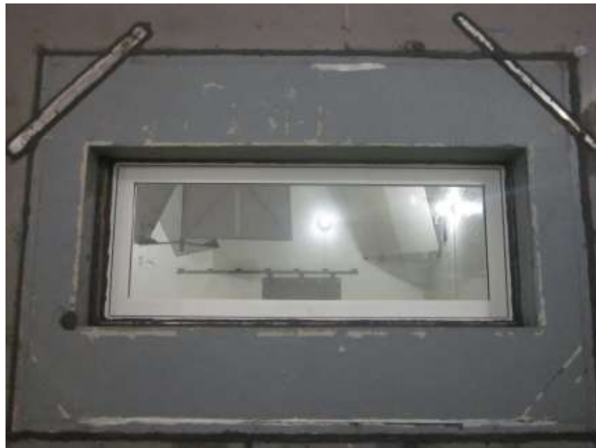
Source Room View of Installed Test Specimen
